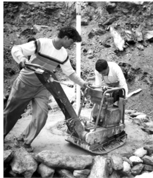
Casing with telescopic coupling being installed in rockfill section of dam, using hand help compactor
