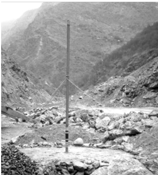
Casing with telescopic coupling installed in rockfill section of dam, supported by guy ropes.
