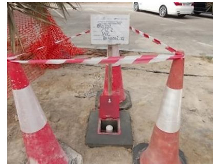
Figure 7-6 Protection for inclinometer
